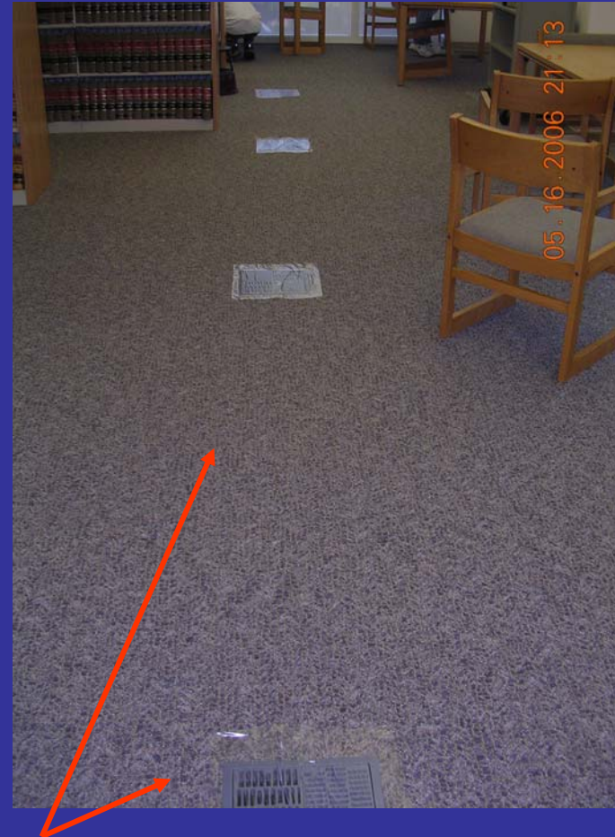
View of Library in FCH-1 with diffusers taped for testing
