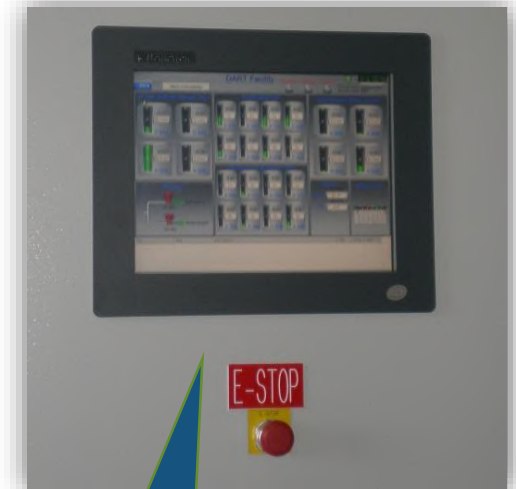
Process Control Panel
